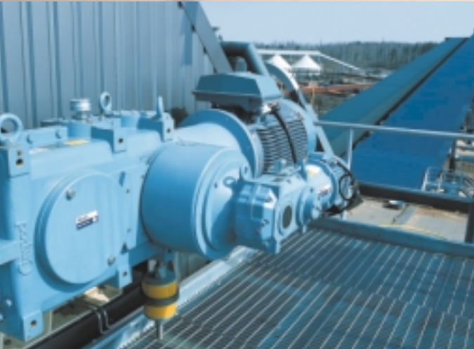
CUMPACT BEVEL GEAR MOUNTED TO A CONVEYOR
